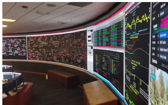
Barco Laser Light Engines add brilliance to the large video wall structure in Evergy's Technical Control Center in Kansas City, Missouri.
