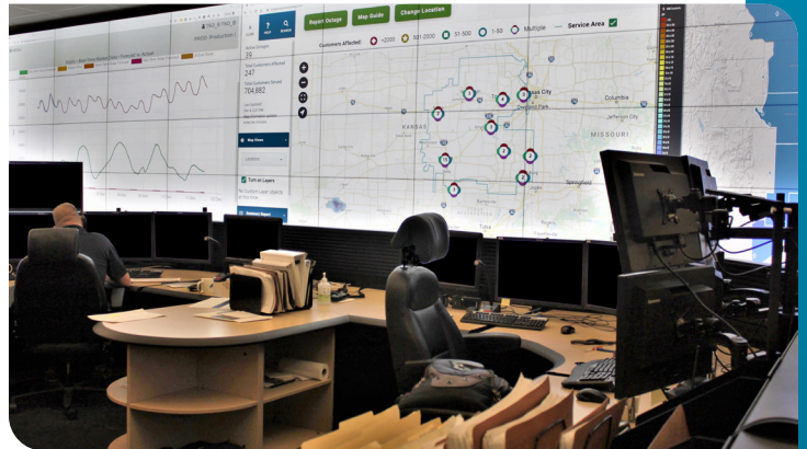
AVI Systems replaced Evergy's large video wall used to monitoring the power company's electrical grid with Barco UniSee LCD panel technology.
